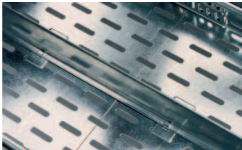
Barrier strip in situ in an MKS cable tray
