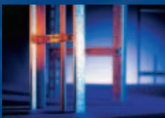
Vertical ladder systems
